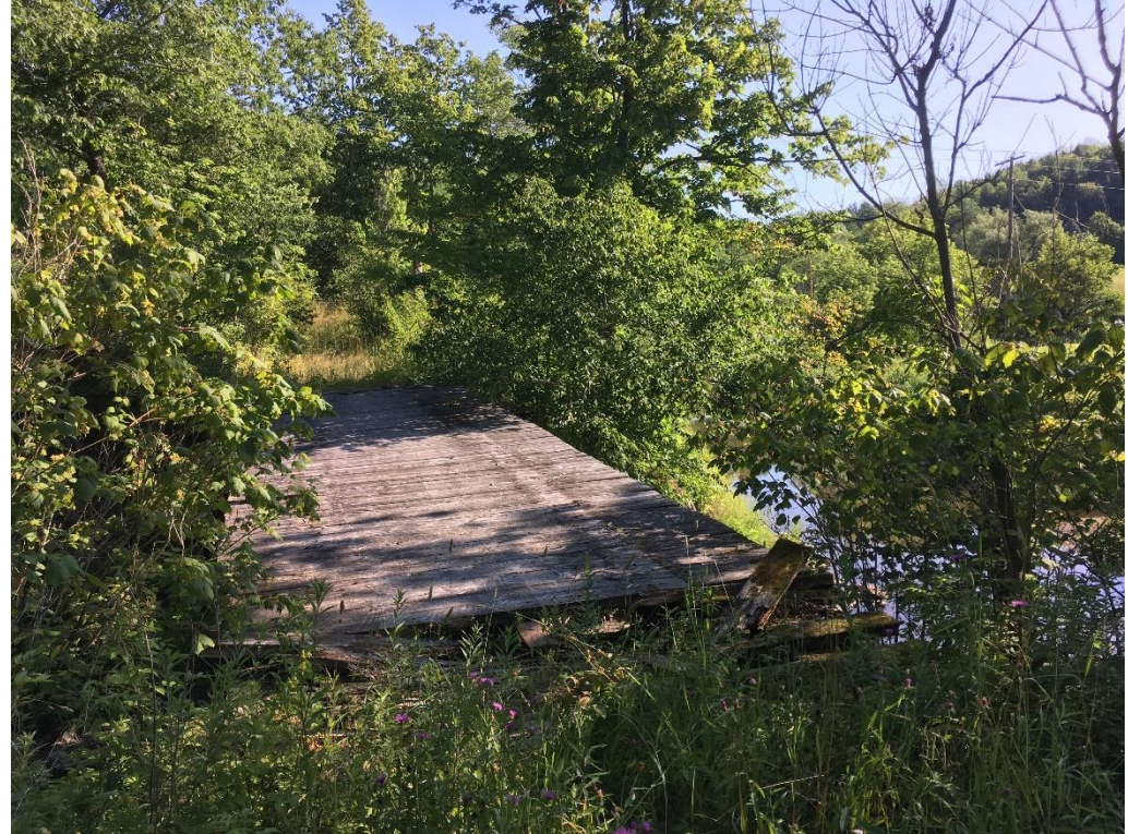
View to north (from rail trail) over bridge deck, 7/24/2019. Note collapsed decking in foreground.
