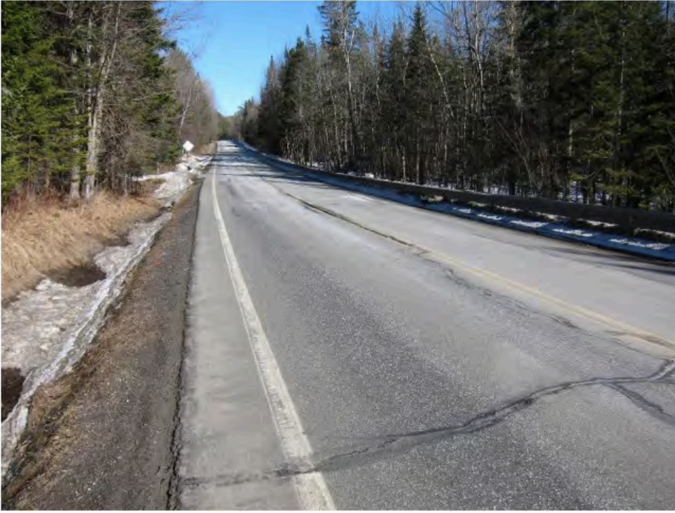
(a) V113 Chelsea-Vershire at about mile 2.60 (centerline tenting on March 7, 2020)
