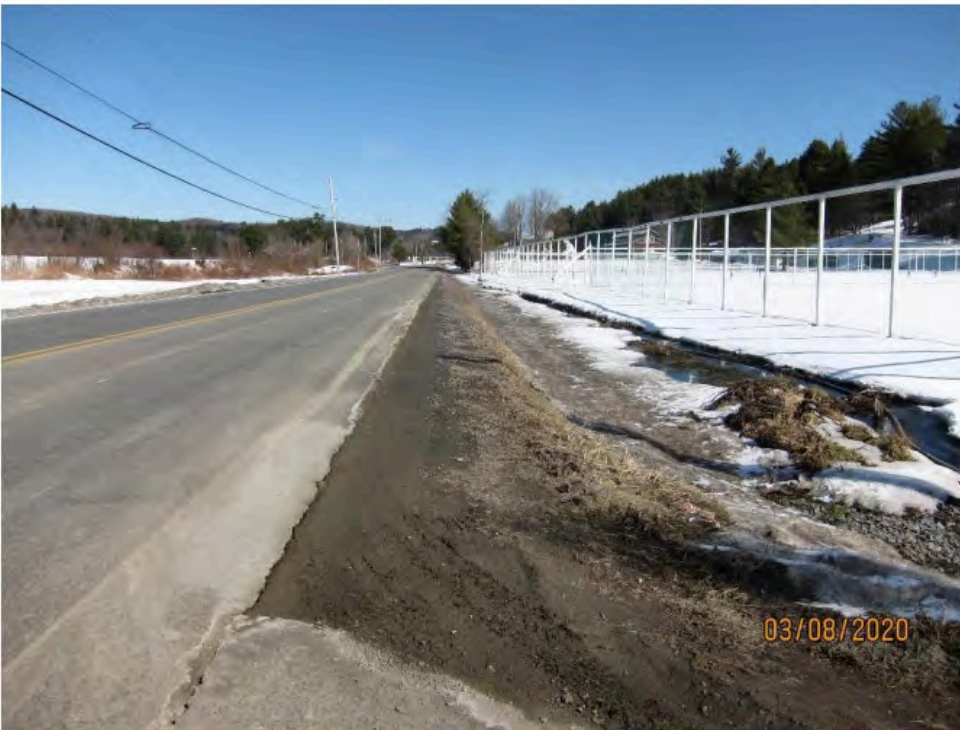
(b) V12A Roxbury-Northfield at Roxbury village (edge heaving on March 8, 2020)
