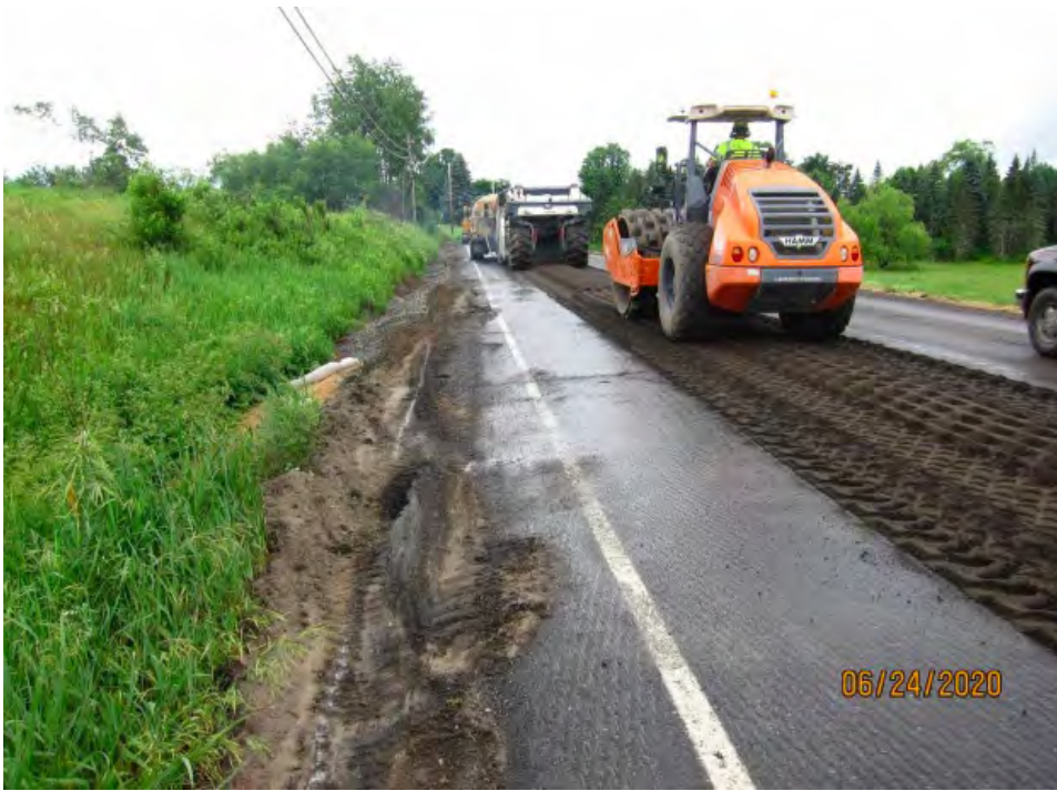
(a) Equipment train with reclaim grinder/mixer supplied by water tanker truck with sheepfoot compactor behind
