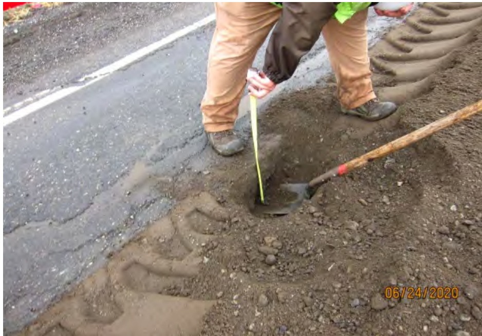
(c) Remaining asphalt beside reclaim pass is about 9 inches thick in this section
