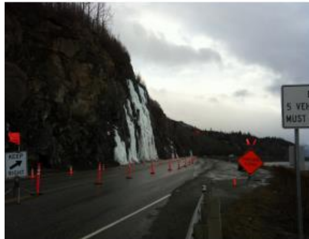
Figure 18 – Traffic pattern modification and detour at MP 113.2 area (Photo by Alaska DOT&PF)
