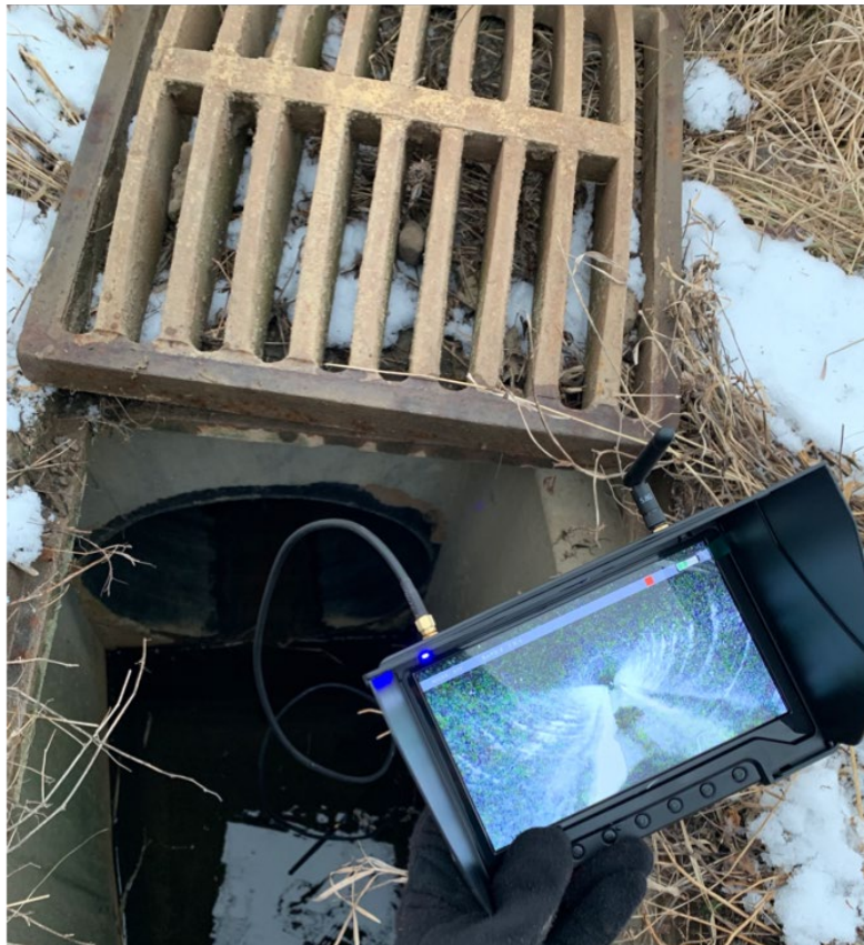
Figure 49 Telemetry Option Test 4 Monitor with antenna placed into line of sight of culvert exit using coaxial extension cable in DI
