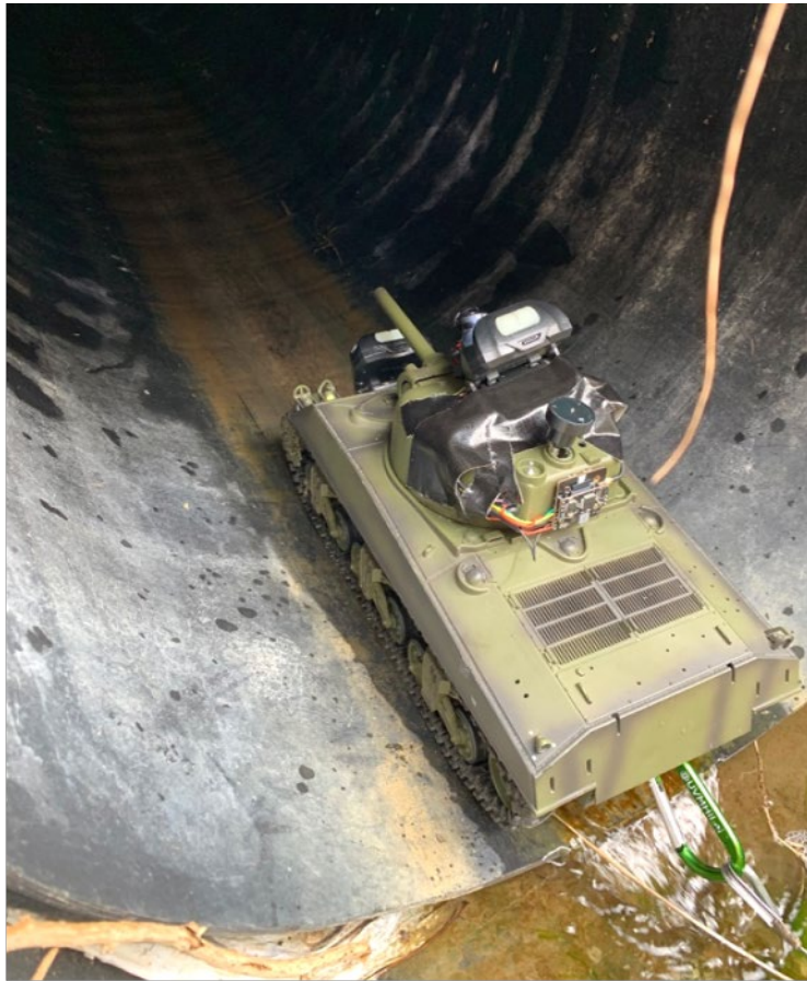
Figure 12 Flowing water in a culvert can be a mobility issue for unmodified HIVE 2.0 tank
