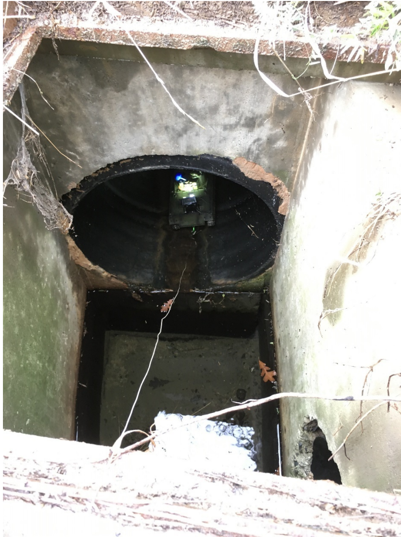
Figure 65 HIVE 2.0 tank at entrance of culvert through drop inlet
