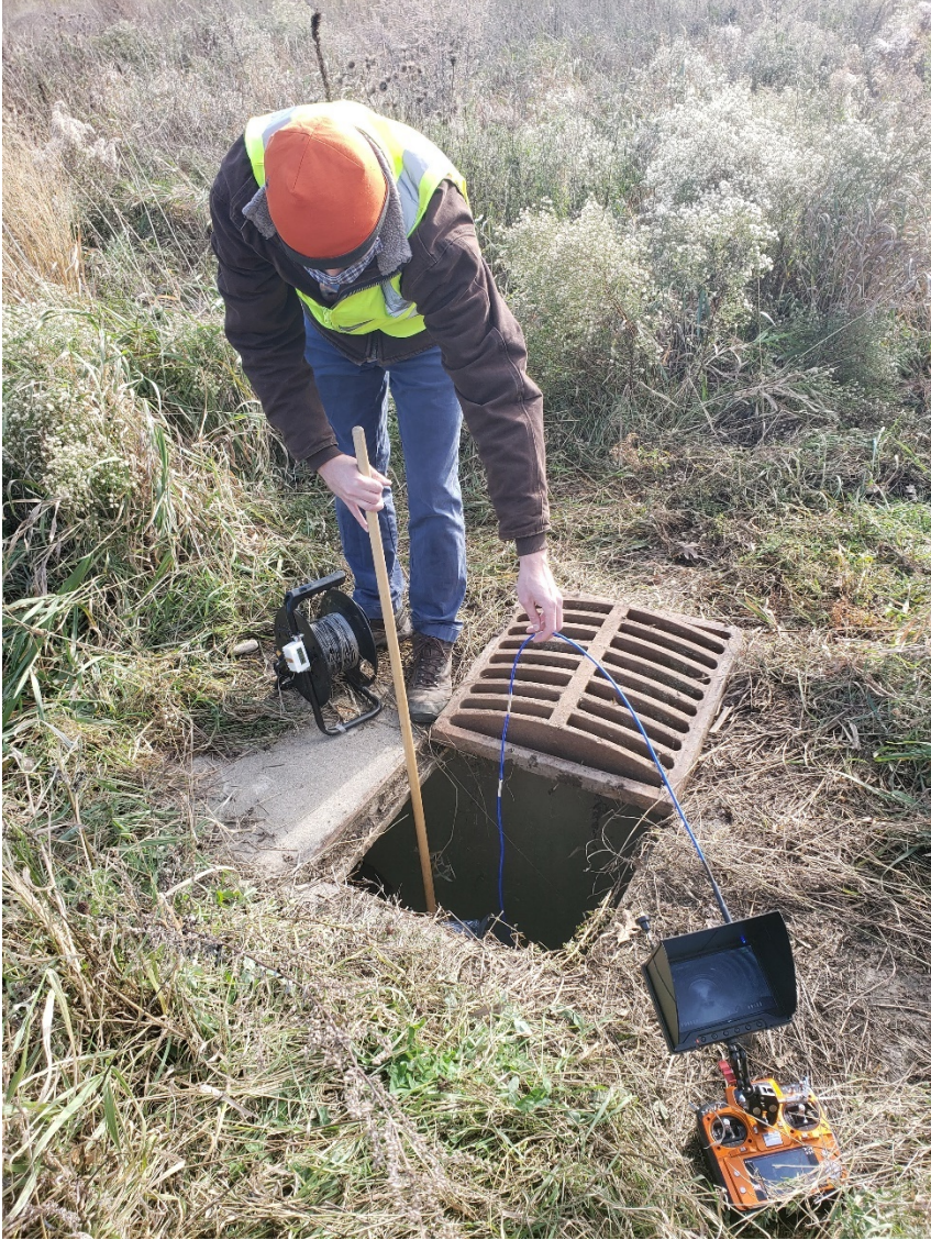
Figure 64 Insertion of video telemetry antenna on extension cable and reflector antenna into drop inlet through utility hole
