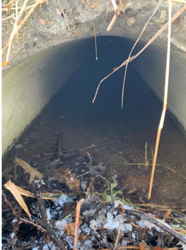
Figure 36. Telemetry Option Test 1 Culvert ID: 64104, 0.457 m (18 inch) diameter, 30.8 m (101 feet) long, concrete, U.S. Route 7, Charlotte, VT
