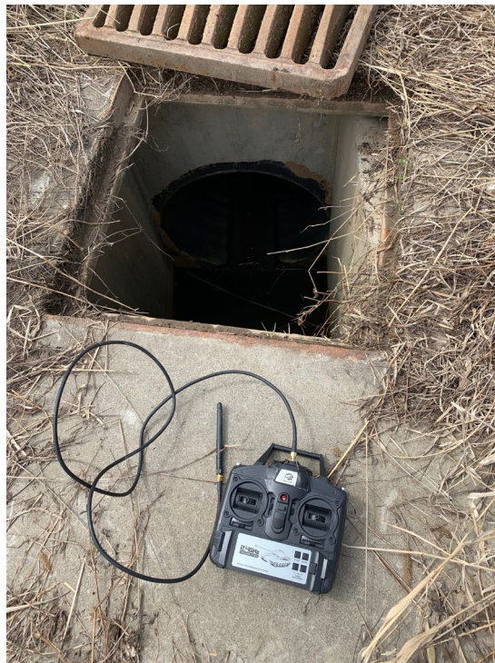
Figure 58 Radio control unit modified with SMA antenna connector and extension cable attached to antenna for possible improved drop inlet telemetry
