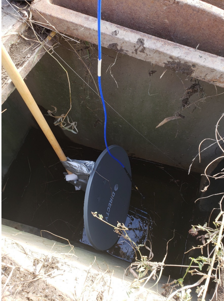
Figure 63 Antenna on extension cable and reflector dish inserted through drop inlet utility hole into telemetry beam line projecting from culvert
