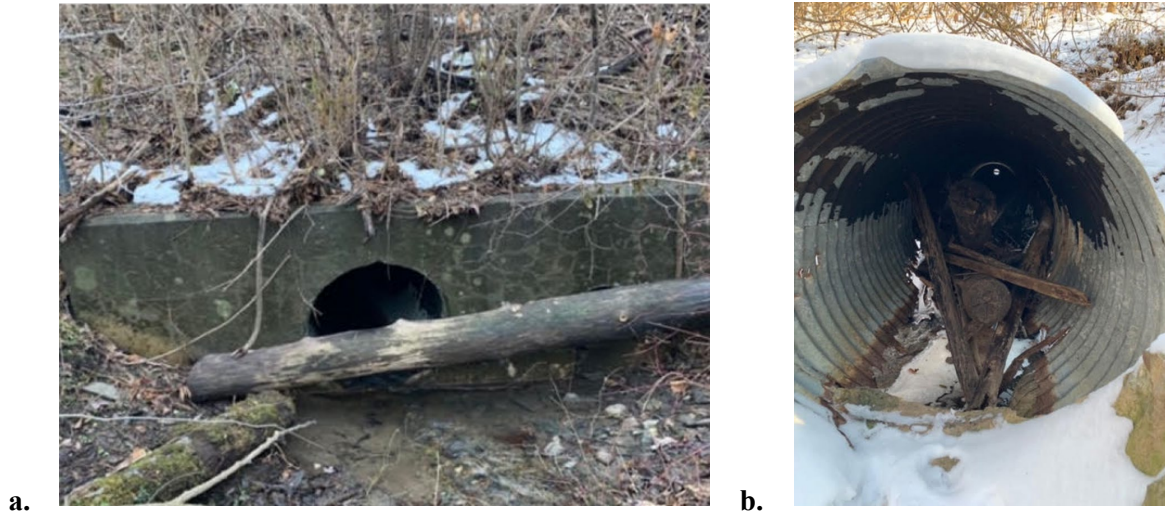
Figure 39. Telemetry Option Test 2 Culvert ID: 64099, 0.762 m (30 inch) diameter, 51.2 m (168 feet) long, metal liner: a. Entrance, and b. Internal debris
