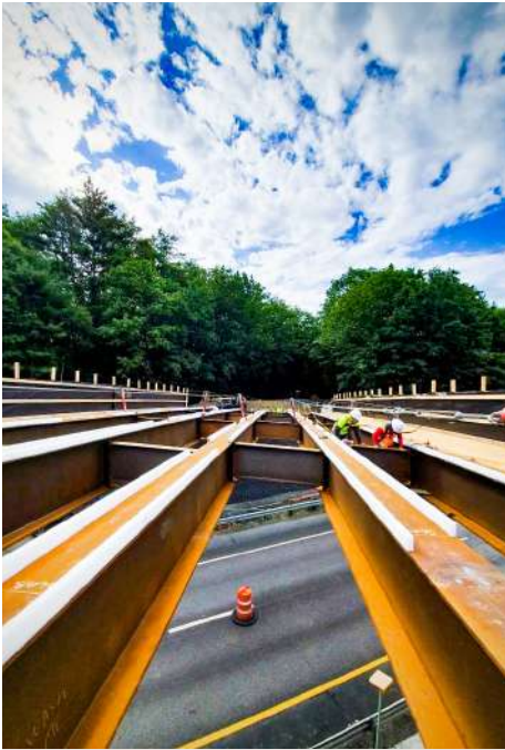
HARTLAND. For high-impact projects, like this bridge replacement over I-91 in Hartland, VTrans sends weekly communications to local stakeholders to keep them informed of the latest construction developments and what to expect on the roadway.
