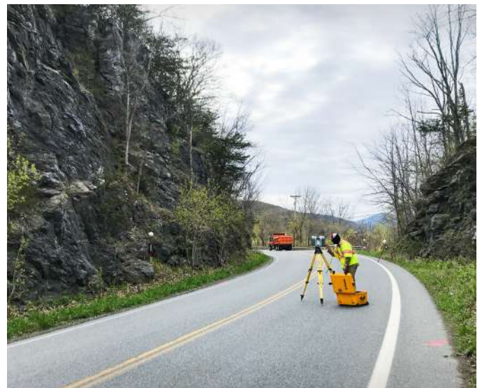
POWNAL. VTrans Survey field crew members use 3D Terrestrial LiDAR scanners to monitor movement in at-risk rock ledges along Vermont roadways. These static laser scanners record light pulses at a rate of one million points per second to create a 3D model of whatever feature or structure is being scanned. Those models are referenced into the Vermont State Plane coordinate system and are used in the design and planning process for transportation projects.
