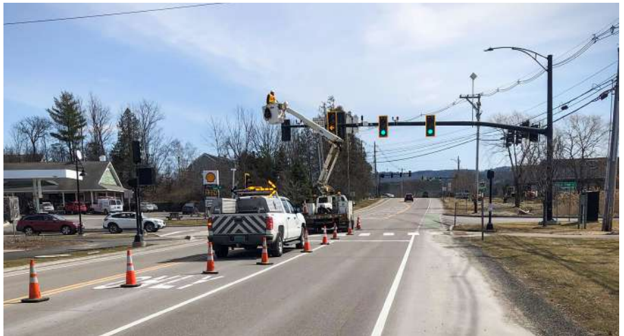
WILLISTON. The steep drop in traffic volumes early in the pandemic created some unique opportunities for different parts of the agency. Slower roadways allowed the VTrans Traffic Signal Unit to safely perform preventative maintenance at some of our busiest intersections.
