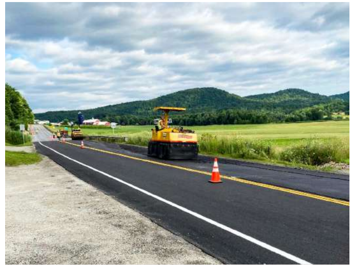
CAMBRIDGE. In 2020, VT-15 was resurfaced from the town of Underhill into Cambridge. This project used an asphalt recycling technique, saving on cost while providing a durable road surface.
