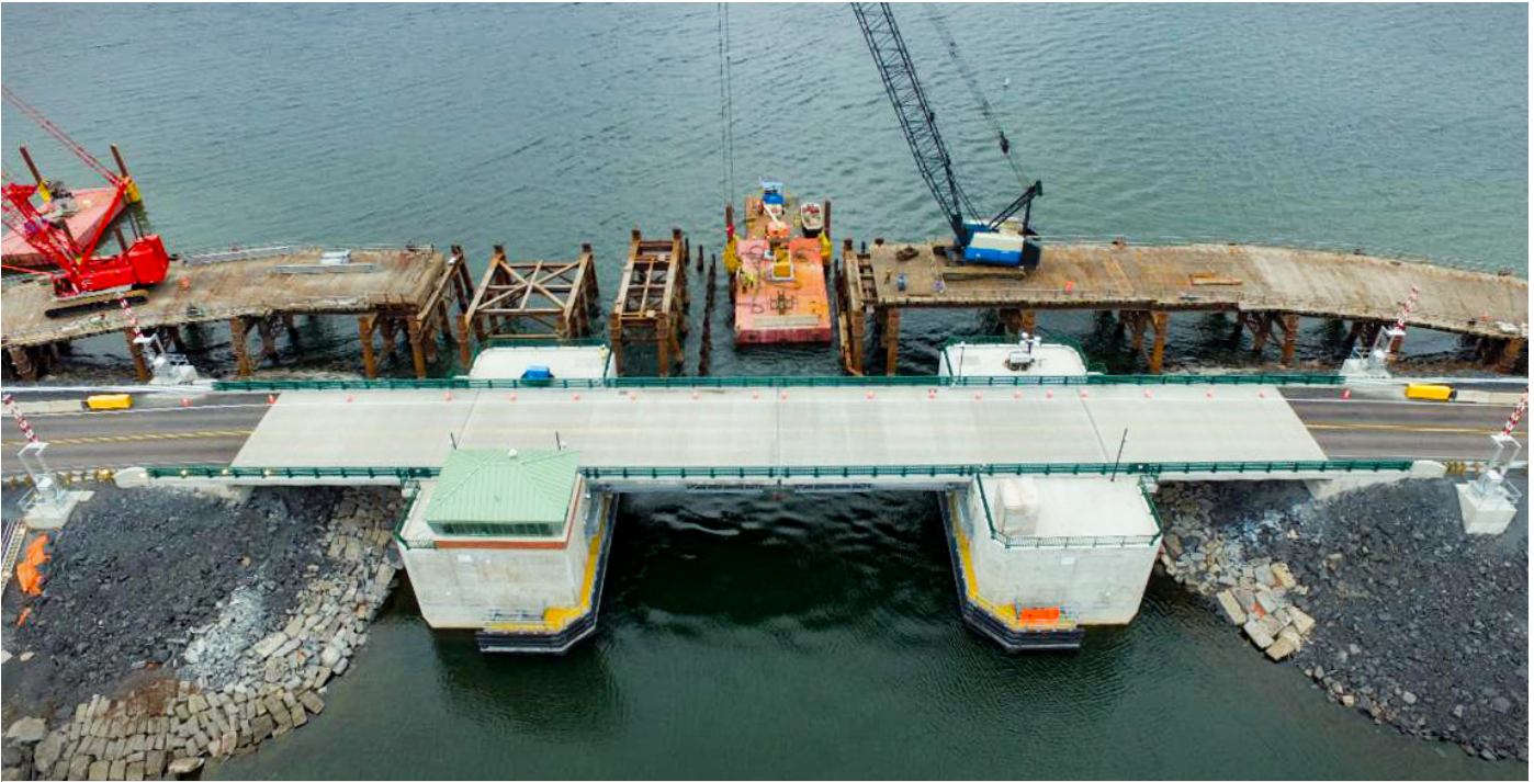
CHAMPLAIN ISLANDS. After many seasons of construction, the new drawbridge connecting North Hero and Grand Isle along U.S. Route 2 was opened to traffic in early November 2022. The new double leaf bascule bridge is the only one of its kind in Vermont and is opened using a combination of electric motors and hydraulics. Comprised of 87,000 pounds of rebar, 6,200 cubic yards of concrete, and more than 15,000 bolts, the new bridge has a design life of 100 years.
