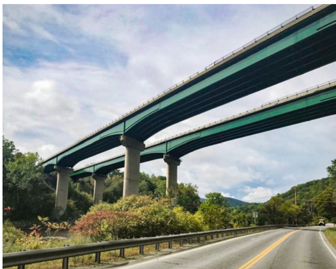
SHARON. Bridge repairs along I-89 over the White River in Sharon were completed this year. Work included rehabilitating both bridge decks with all structural steel stripped and recoated.
