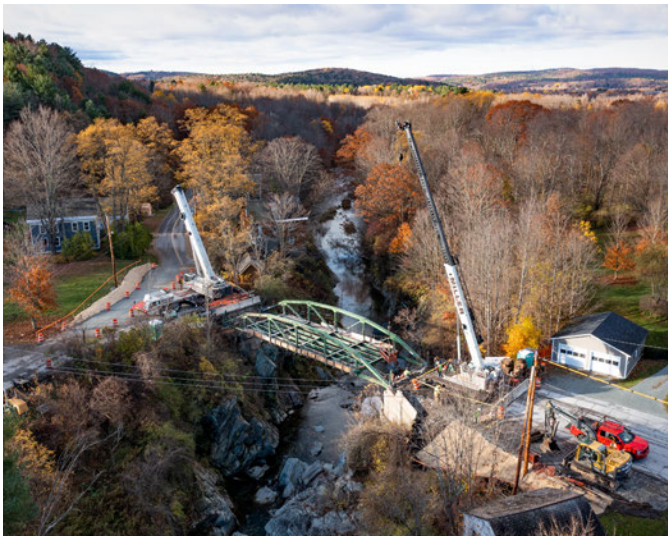
POULTNEY. The historic truss bridge over the Poultney River proved a challenge to move. Cranes were required on both sides of the bridge in order to safely elevate and relocate the structure to the north side of the chasm for disassembly while avoiding contact with neighboring homes and utilities.
