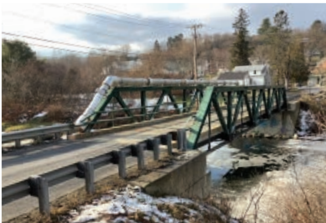
INDEFINITE DELIVERY/INDEFINITE QUANTITY CONTRACTING. ID/IQ was utilized for one State highway bridge project and one town highway bridge project in 2019. The Bradford bridge project on Creamery Road included a deck replacement for the historic pony truss. The project had a limited scope to replace the existing failed FRP deck with a half-filled concrete steel grid deck. The Hinesburg project on VT Route 116 involved the replacement of the existing cattle pass with a new 78-inch diameter polymer coated corrugated steel pipe.
