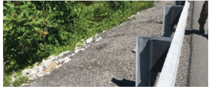
PROCTOR. Simple erosion control fixes, like this one along US-4, have a demonstrable effect on improving water quality.
