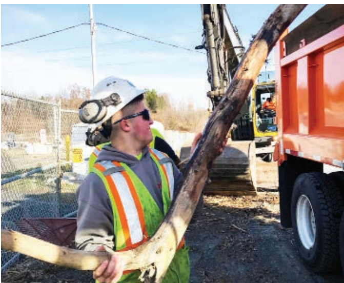
STATEWIDE. Flooding from the Halloween rainstorm closed more than 20 state highways. Crews from different regions teamed up and worked tirelessly to repair the damage.
