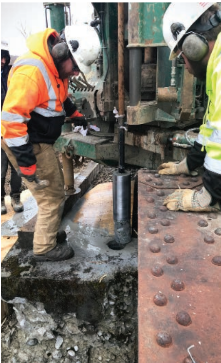
COVENTRY. All VTrans construction projects require proper planning and usually bring together diverse parts of the agency. An upcoming rail project gathered Rail, Geological, and Materials crews to collect core samples for close inspection.
