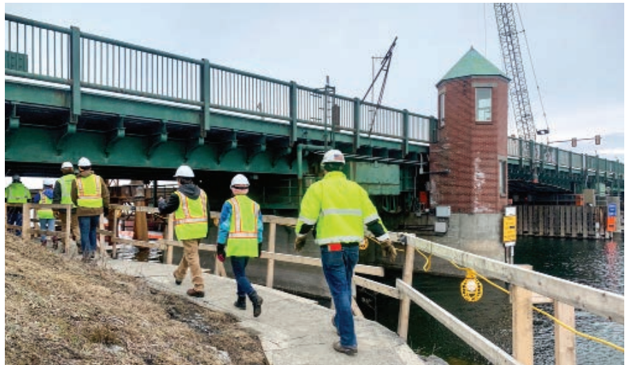
NORTH HERO - GRAND ISLE. Supporting STEM education is essential to the Agency's goals. Playing host to class trips on sites like the North Hero/Grand Isle Drawbridge replacement project is a great way to expose students to engineering in action.
