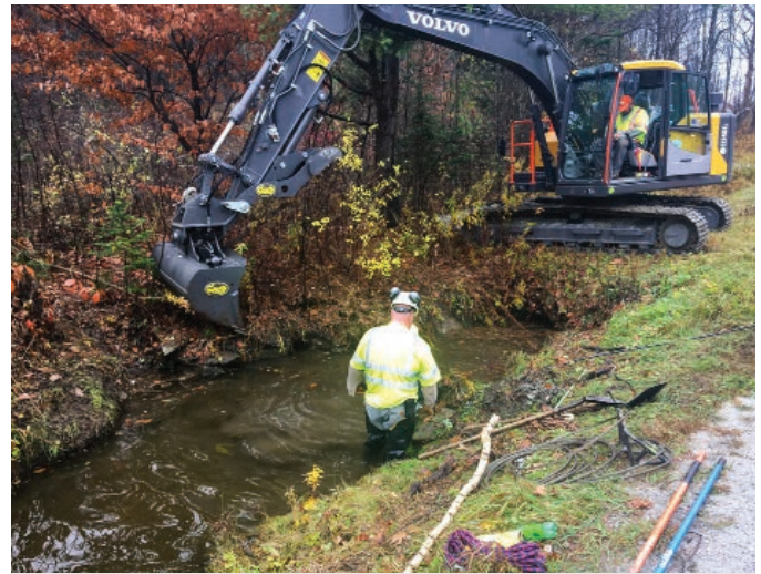
STATEWIDE. With thousands of culverts in our highway network, maintenance crews work year-round to keep them flowing and clear of debris.
