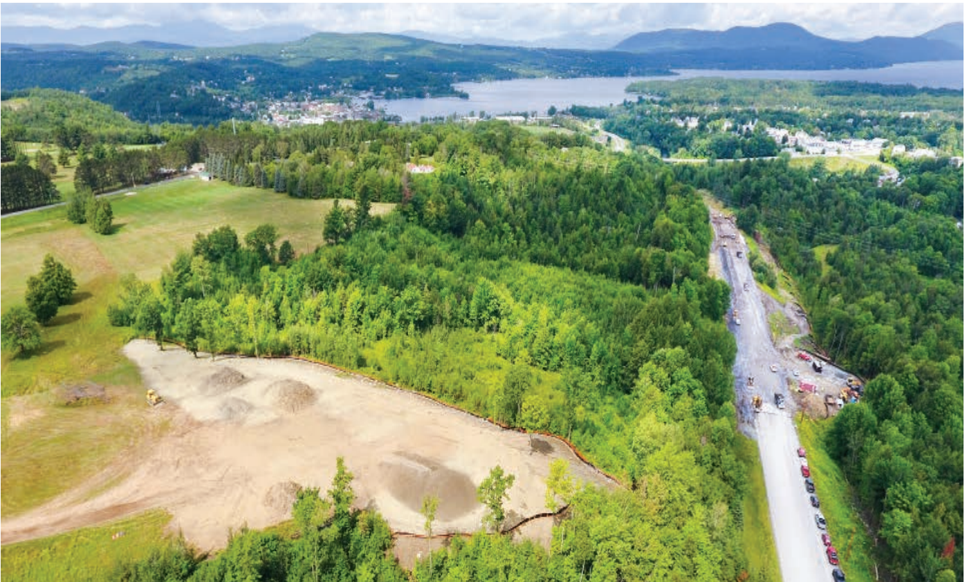
NEWPORT CITY. Remediating slope failures along VT-191 required full-depth reconstruction of the roadway, replacement of a failed culvert, and installation of three active wells to extract water from below the road surface.
