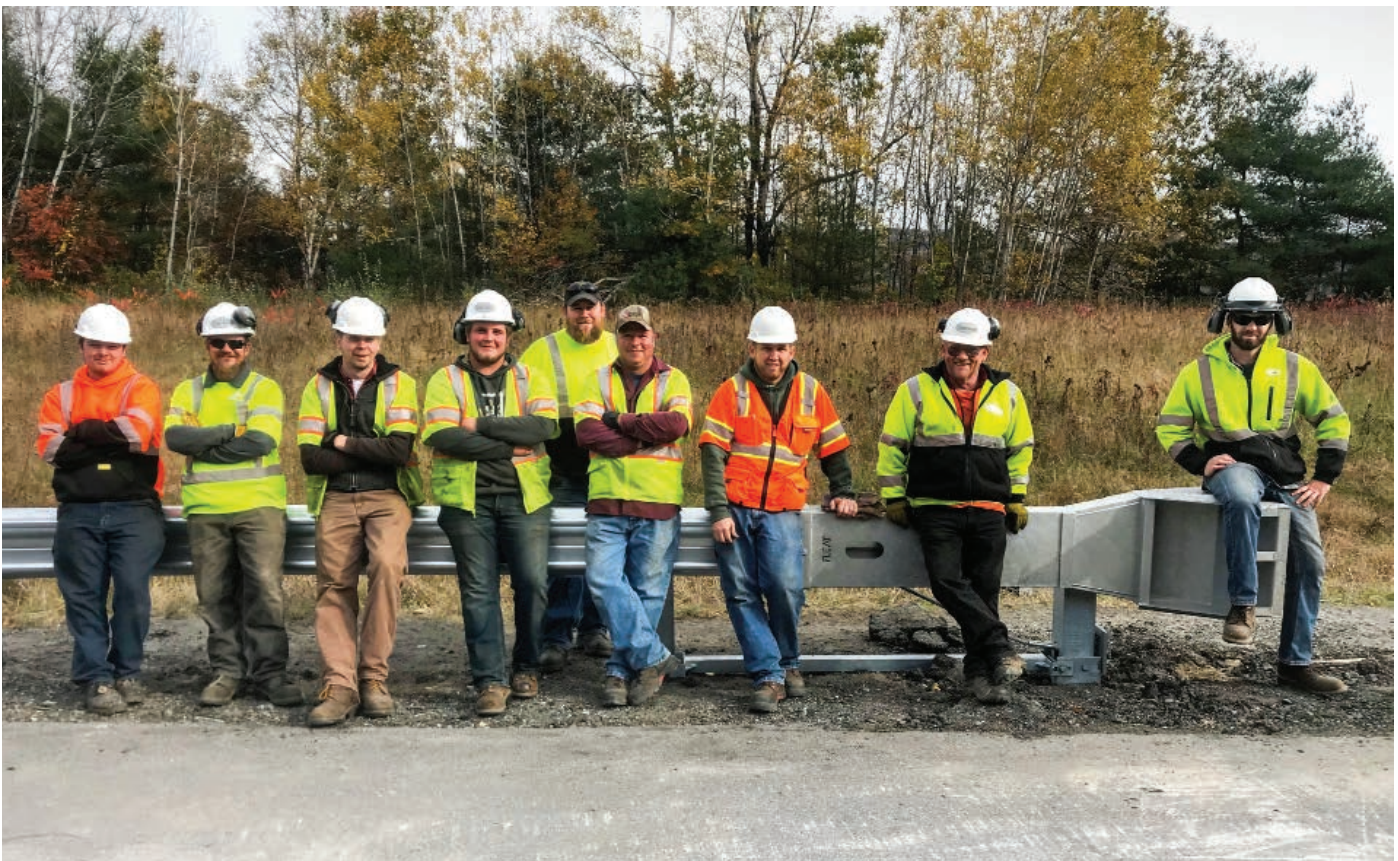
Crews from Thetford and Williamstown teamed up to install a new guardrail terminal end system, the first installation of its kind in the United States. These new systems will be replacing old ones throughout the state, increasing durability and safety while decreasing long-term costs.
