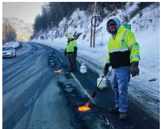
GROTON. Pothole patching can be an effective temporary fix but often requires a little heat in colder months to help the material stick to the road surface.
