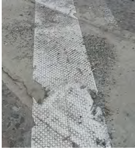
Figure 14: Tape wear over the higher points on the TechCrete repair
