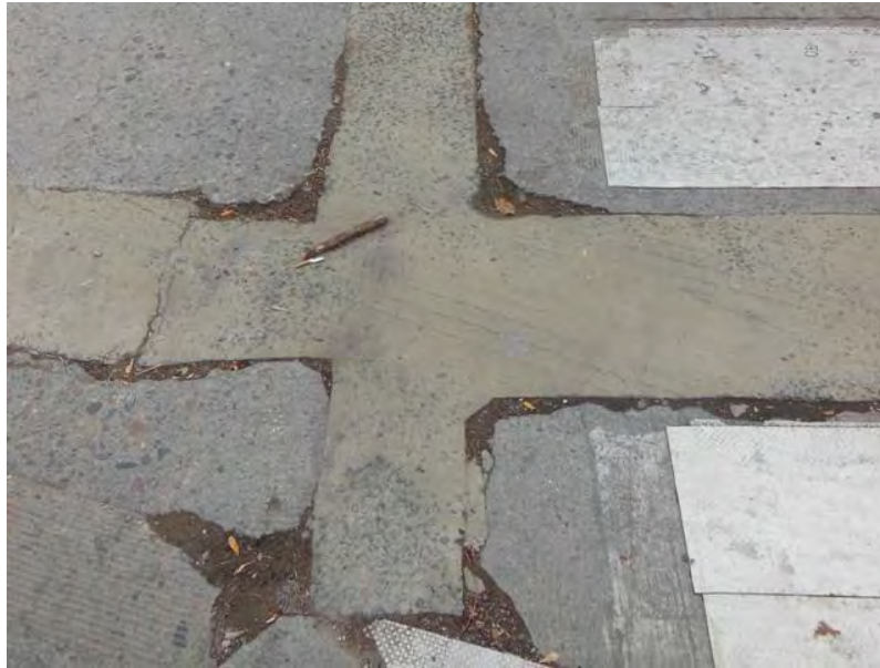
Figure 16 Condition of some repair areas following the fourth winter of service life (2013).
