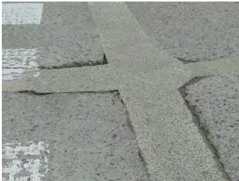
Figure 15 Condition of some repair areas following the second winter of service life (2011).
