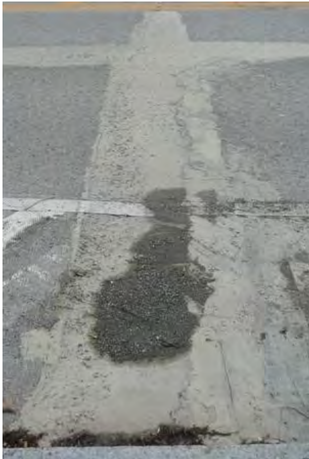
Figure 12: Condition of joint following first winter season
