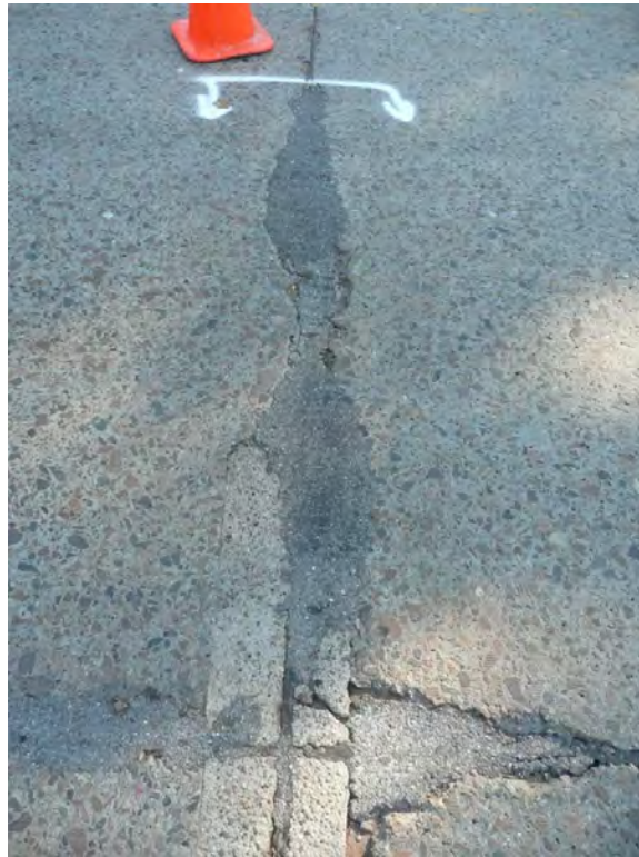
Figure 4 Typical concrete joint deterioration prior to repair
