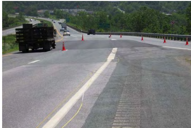
Figure 5.2 Interstate 89, Hartford, Vermont looking east toward New Hampshire. The asphalt patch extending across both southbound lanes indicates the region of subsidence.
