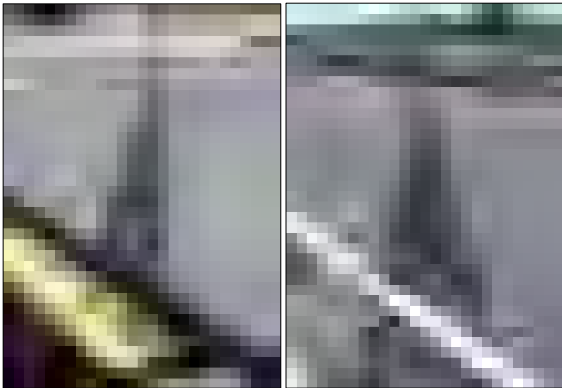
A) Finger Expansion Joint (north)
