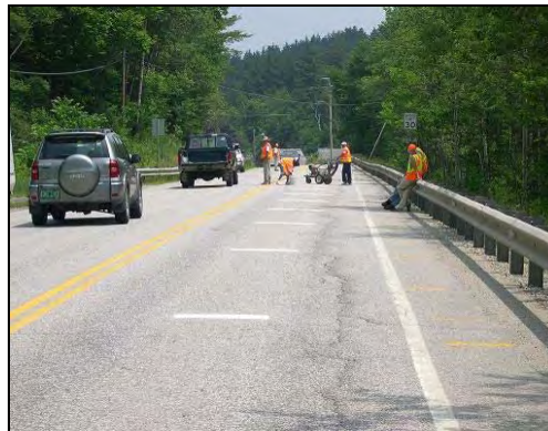
Figure 3 – First Year Installation
