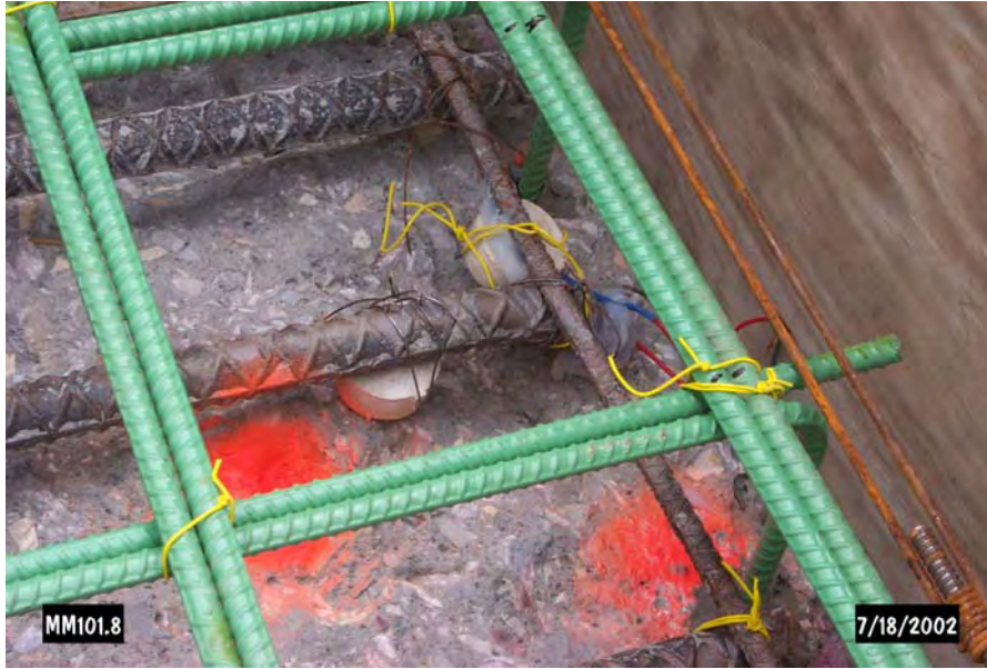
Galvashield XP Anode and Test Kit installed in the Cap of Pier 2 on Br. 48N
