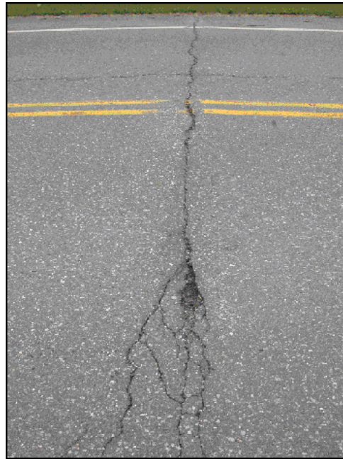
Figure 12–Crack 9m south of edge, 2007
