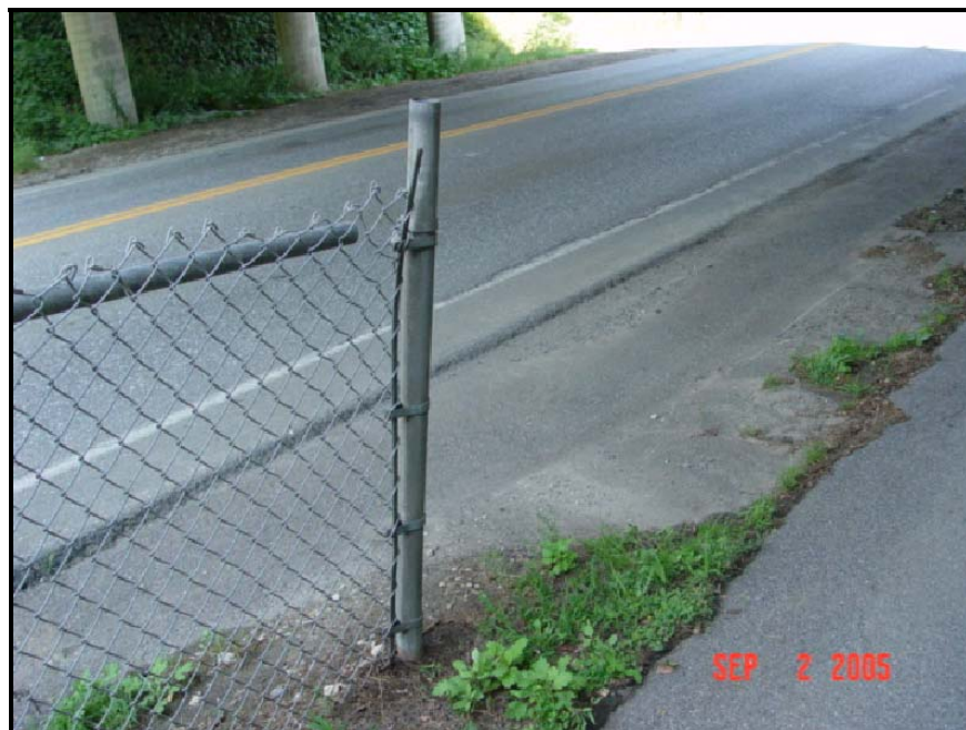
Figure 52: South Burlington - Inconsistent Use of Fencing
