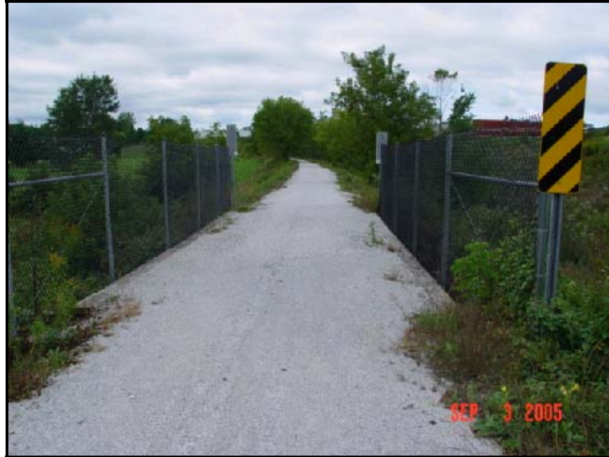
Figure 28: Missisquoi - Cattle Chute Effect from Chain Link Barriers on Each Side of Path
