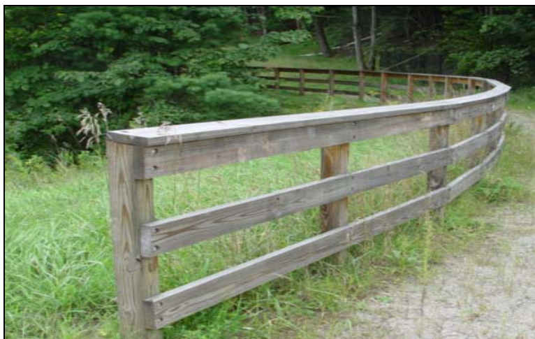
Figure 16: Wood Safety Railing
