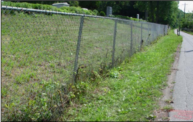
Figure 18: Plain Chain Link Fence
