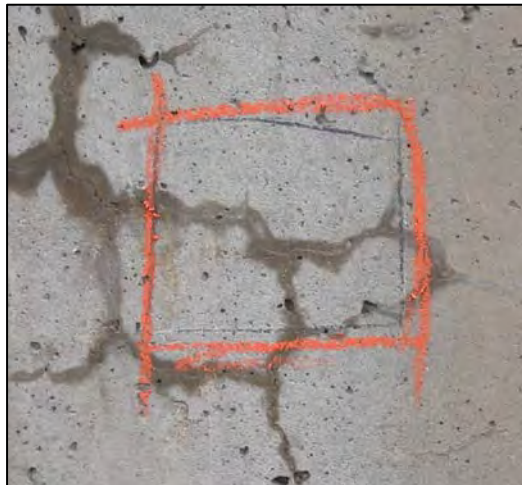
Figure 1 Crack with white precipitate.
