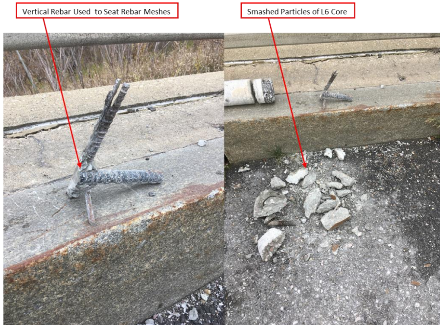
Figure 12: Photos of a Vertical Rebar Found within L6 Core. It's a Mesh Seat Used to hold the Rebar Meshes in Place During Construction.
