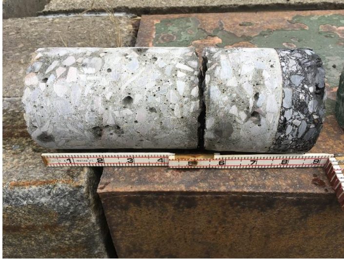
Figure 10: Area 1, L5 4in Core. Cannot Be Seen in the Image but Had 2 Rebar Meshes were Present.
