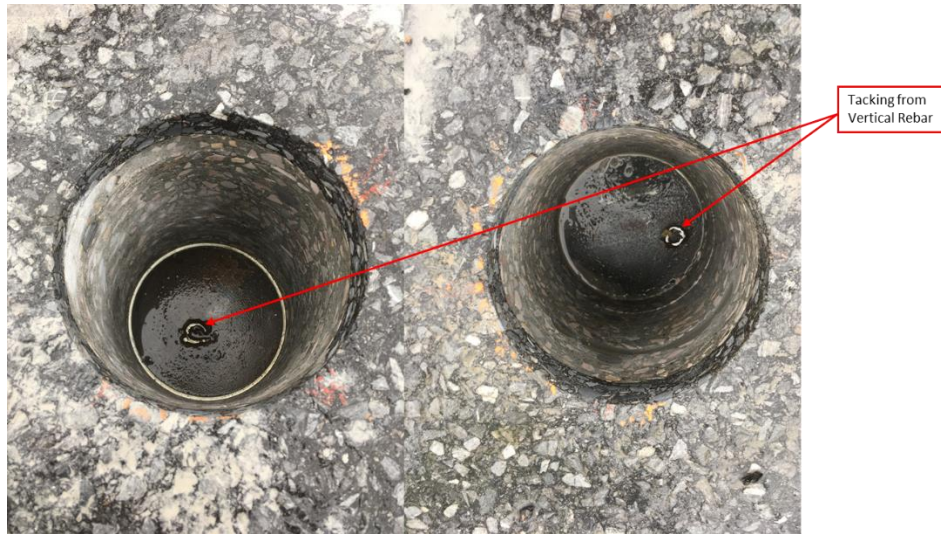
Figure 20: Coring Holes from Area 2, L1 (Left) and L3 (Right). Tacking Material from the Vertical Rebars can be Seen on the Top Surface of the Steel Girder.
