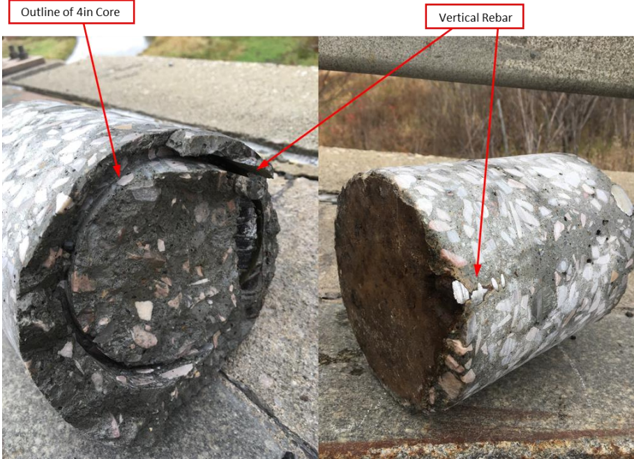
Figure 11: Area 1, L6 6in Core. Vertical Rebar was Present Which Can Be Seen in Both Images. A 6in Core had to be cut Around the 4in Core Because the Drill Bit was Cutting into the Vertical Rebar.
