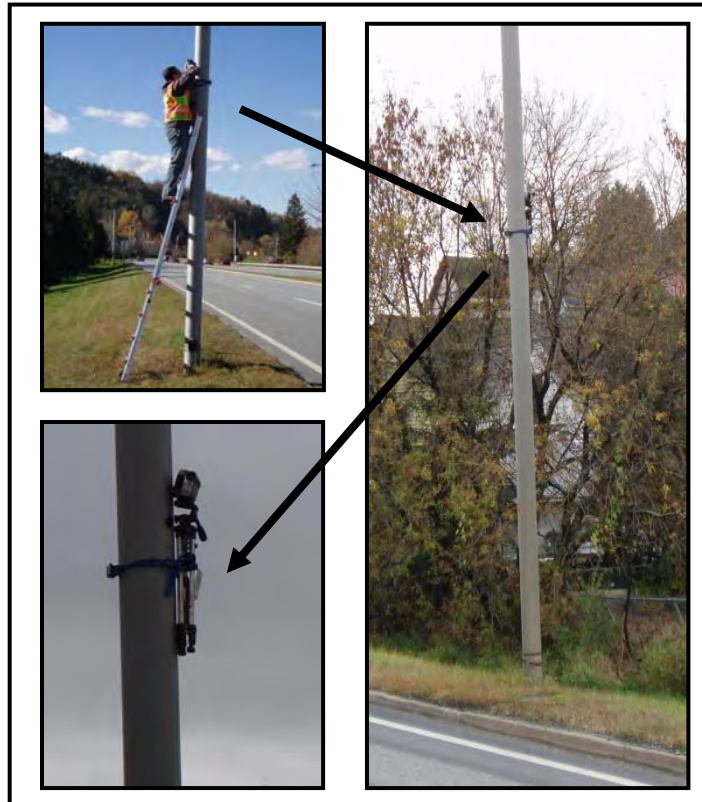
Figure 13 Example of Typical Video Camera Installation
