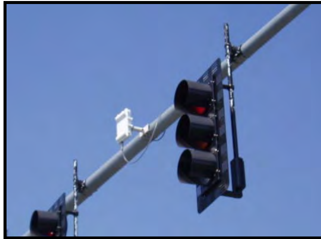
Figure 26 Installation of the SmartSensor in Vermont
