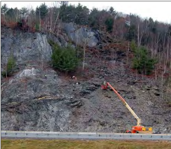
Figure 11 Preparing Slope for Hybrid System Footprint and Excavation for Steel Post Foundation Pads.
