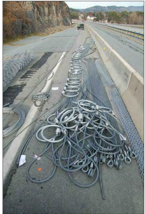
Figure 5 Support Cables, Breaking Elements and Rope Anchor Cables.
