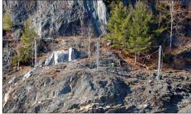
Figure 13 Lacing Support Wire Ropes.
