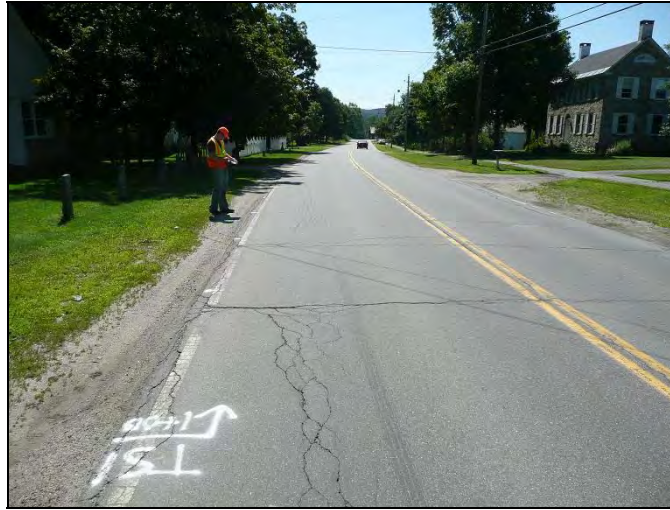
Figure 4. Typical Fatigue Cracking
