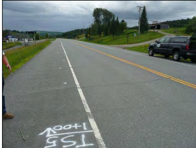
Figure 7. Typical Thermal Cracking
