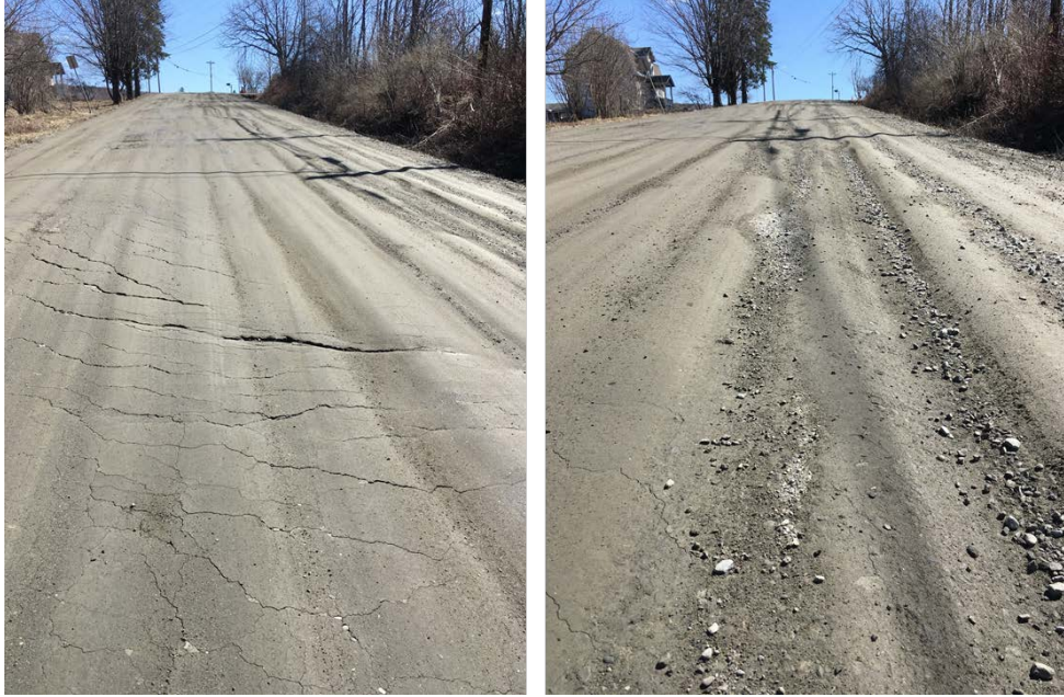
Figure 12: Stone Road Near Intersection with VT 64 on a Hill (Town Road with no RAS). Road cracking, rutting, depressions and potholes were widespread. Photos taken during 4/14/17 Site Visit. See also Stone Road video .
