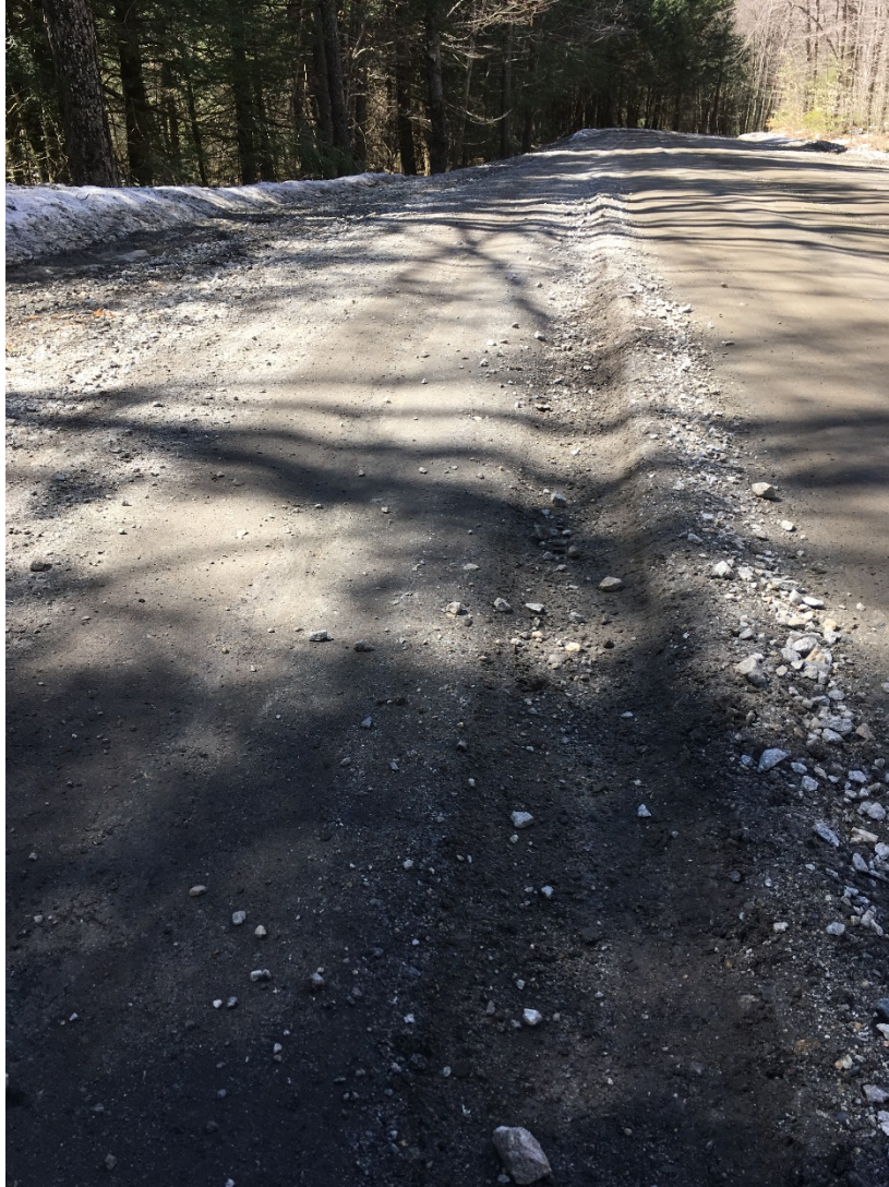
Figure 11: VT 65 Looking Down Decline Towards VT 12 Mile Marker 0.8. Some Rutting is occurring on the left side of the road. Photo taken during 4/14/17 Site Visit.
