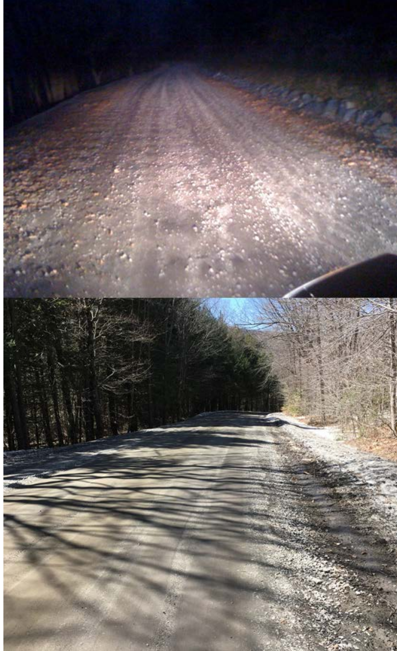
Figure 5: VT 65 Looking Down Decline Towards VT 12 Mile Marker 0.8. Photo Comparison between 10/26/16 Site Visit (Top) and 4/14/17 Site Visit (Bottom). Minor ruts formed on the left side of the road and can be seen in more detail in Figure (11)
