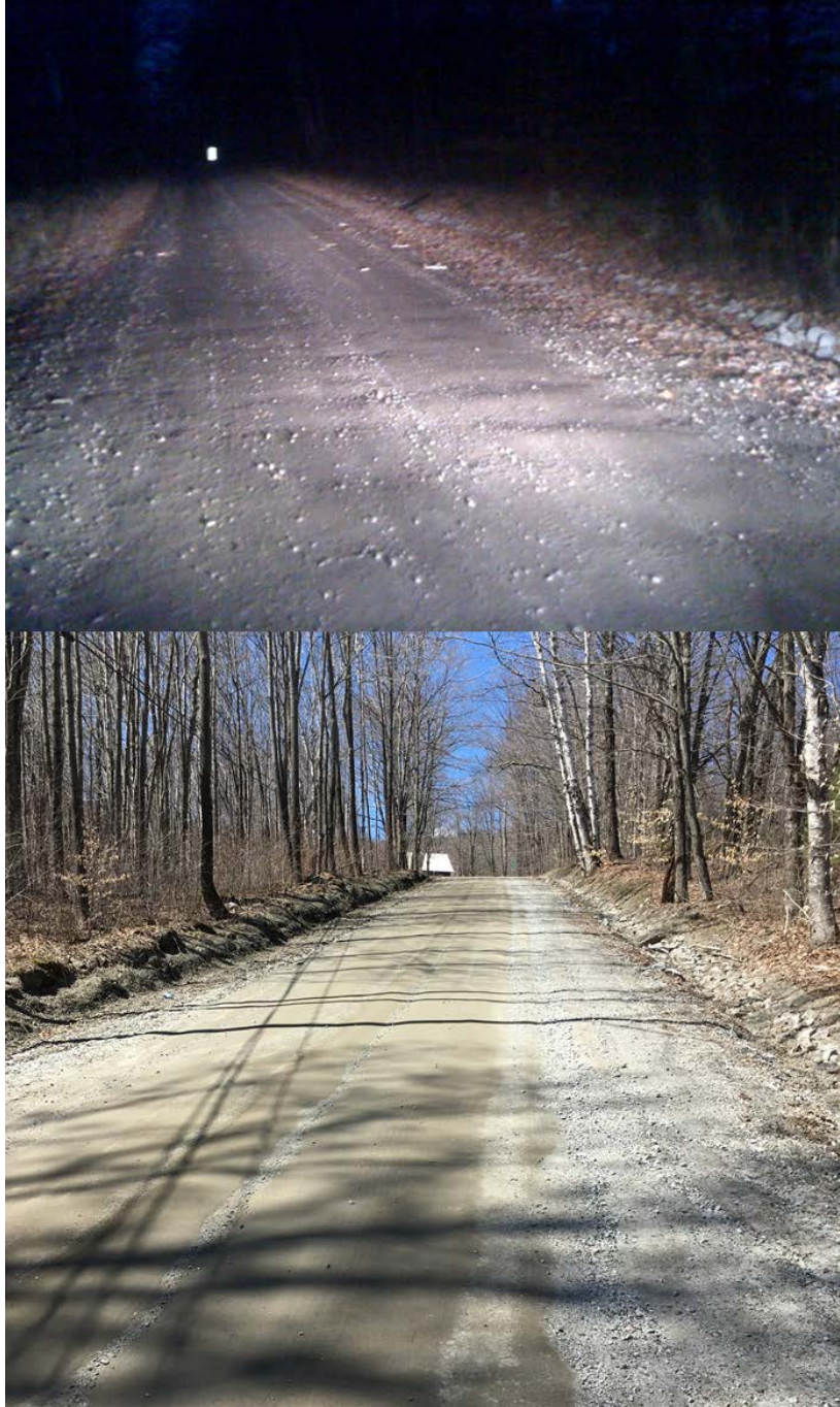
Figure 3: East of Intersection with Bear Hill Road at VT 65 Mile Marker 2. Photo Comparison between 10/26/16 Site Visit (Top) and 4/14/17 Site Visit (Bottom)
