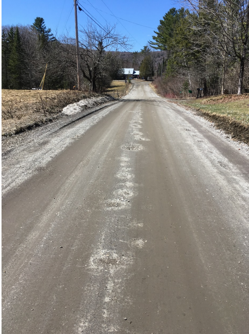
Figure 10: VT 65 just West of I-89 Overpass, Mile Marker 2.7. Photo taken during 4/14/17 Site Visit.
