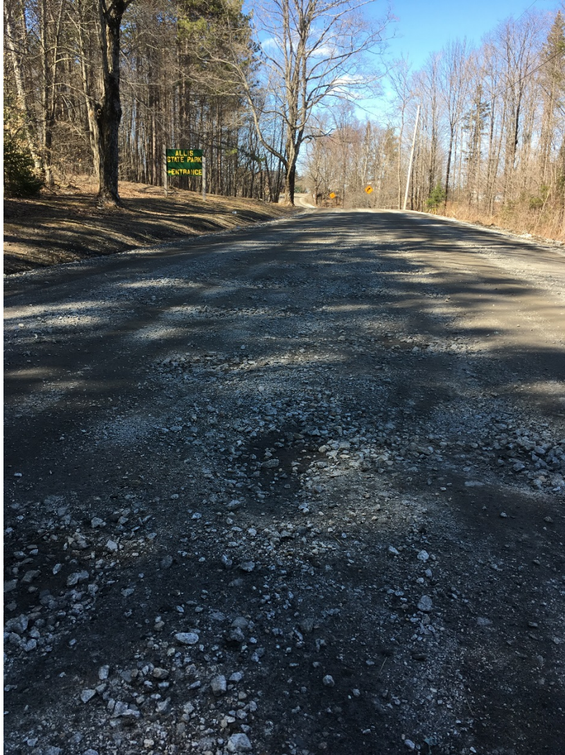
Figure 9: Potholes Near the Entrance to the Allis State Park, VT 65 Mile Marker 1.4. Photo taken during 4/14/17 Site Visit.
