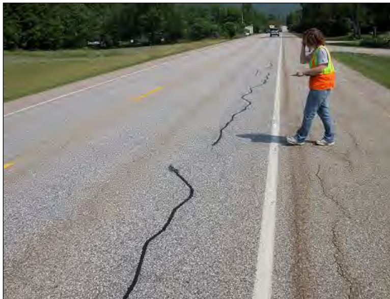
Figure 6 Fatigue cracking (Test Site 2, year 10)
