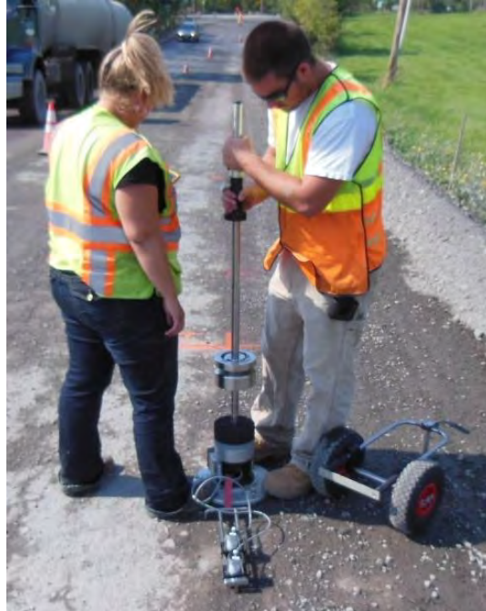
Figure 4 Light Weight Deflectometer (LWD) being used to collect data on a project.
