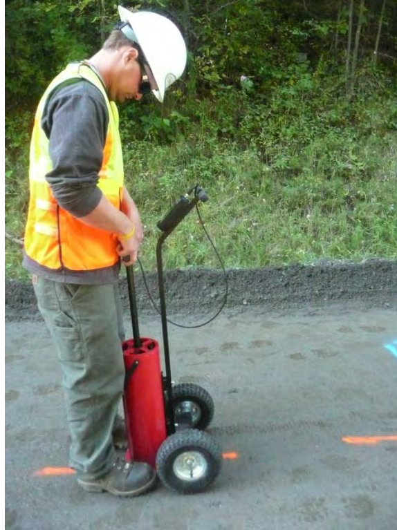
Figure 3 Clegg Impact Soil Tester (CIST) being used to collect data on a project.
