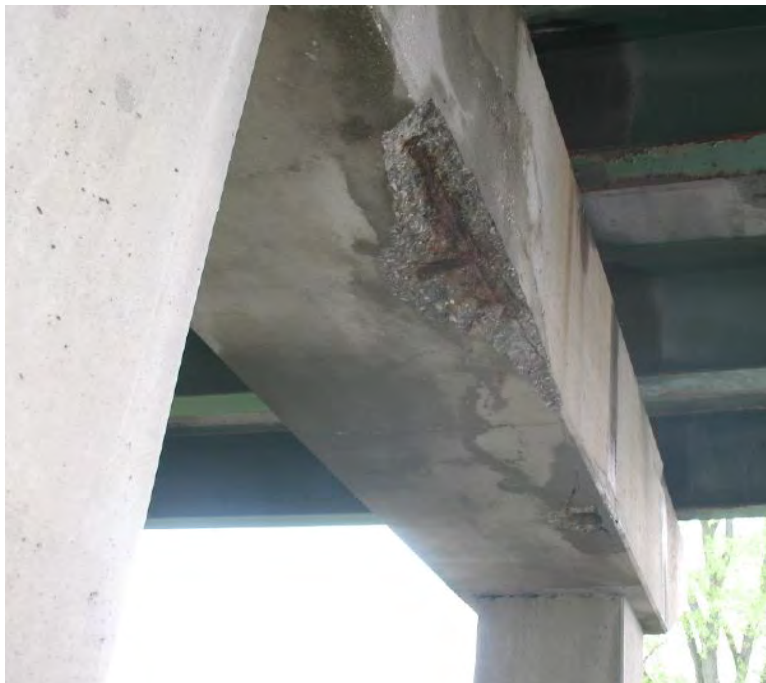
Figure 3 Concrete distress in pier bent (VTrans 2010)
