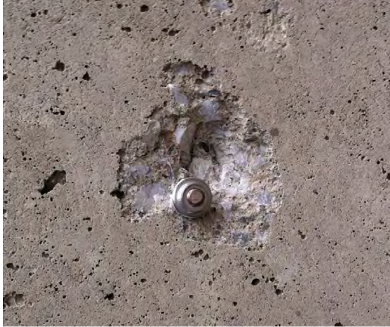
Figure 7 Powder Actuated Faster Caused Concrete to Burst (VTrans 2014)
