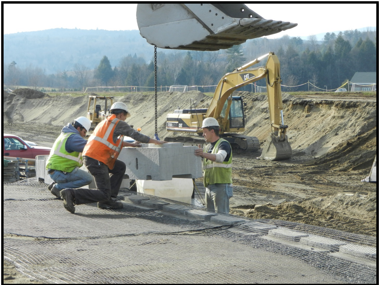
Figure 1: Segment of the ReCon wall illustrating the interlocking keys cast into the blocks and geogrid reinforcement to be embedded into the soil
