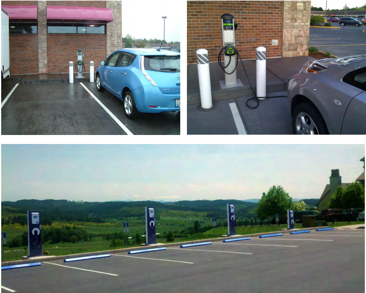
Figure 7.1: Photos of Typical EVCE Stations
