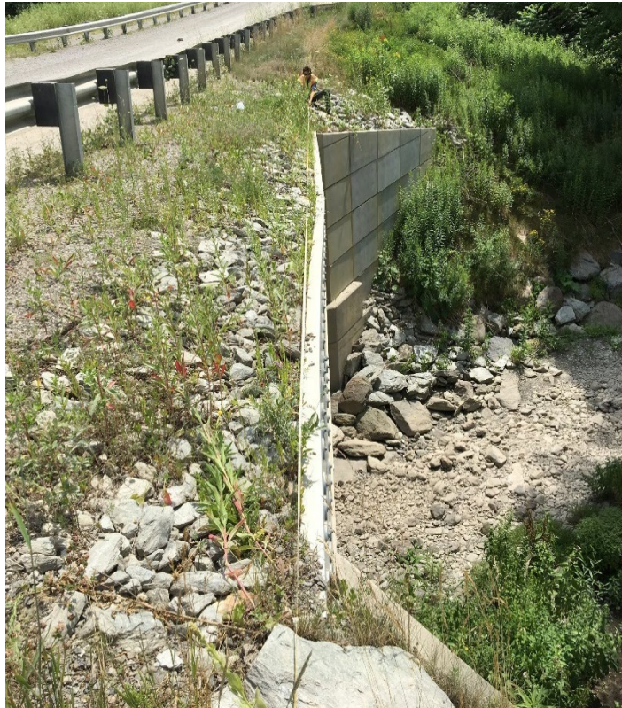
Figure 16: Bowing on Western Headwall
