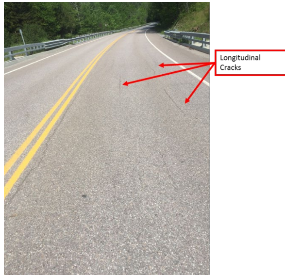
Figure 9: Longitudinal crack on northbound lane (June 2, 2016)
