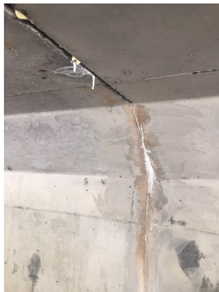
Figure 11: Bridge underside deposits (June 2, 2016)
