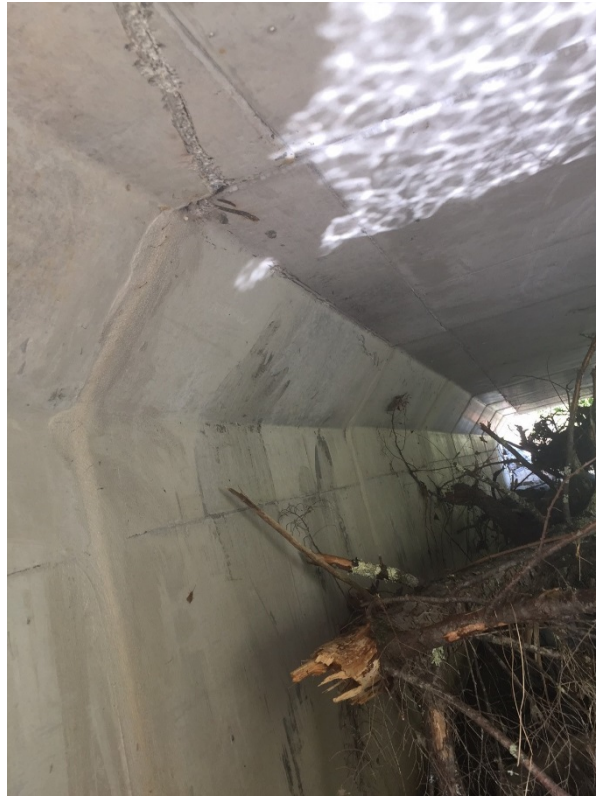
Figure 19: Underside with debris (August 15 ,2017)
