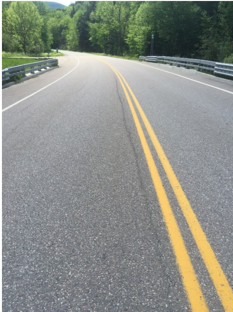
Figure 7: Centerline crack throughout bridge (June 2, 2016)
