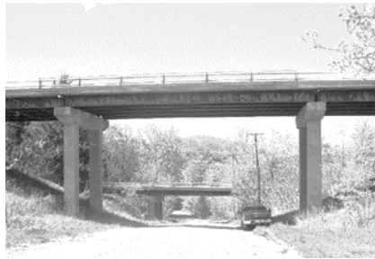
a) Bridge A with a two square column bent at 30-ft-tall supporting simple span multiple beams
