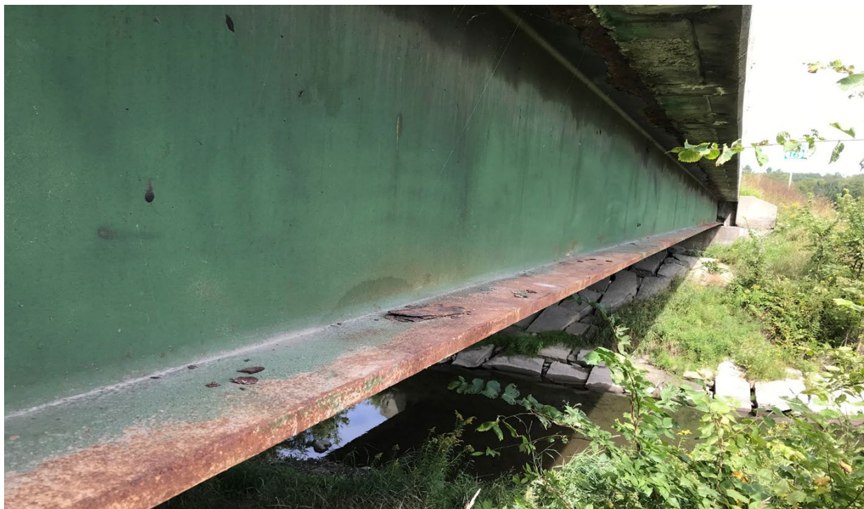
Hardwick VT Br. 1 (Fascia beam paint deterioration)
