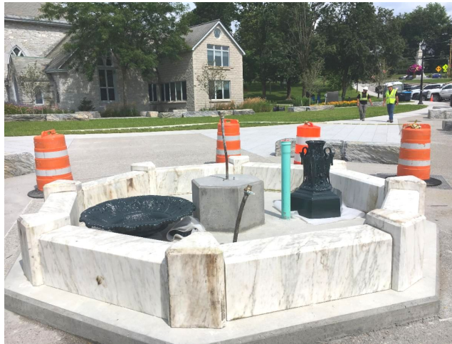
The above photo shows progress on the fountain in Triangle Park. It is anticipated to be turned on during the dedication ceremony on August 21, 2021.
