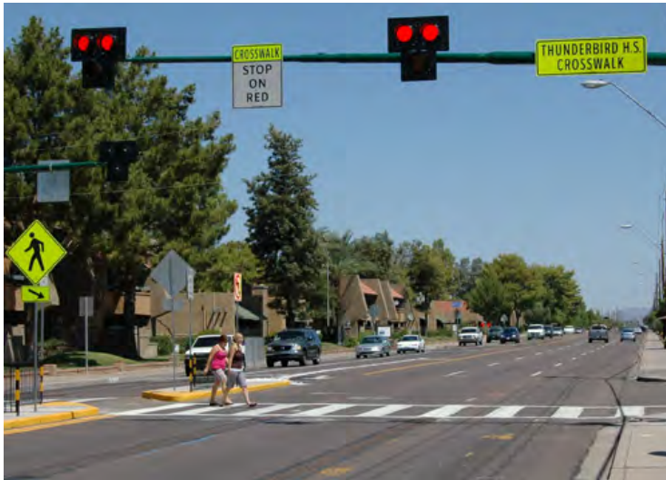
Typical installation of Pedestrian Hybrid Beacon
