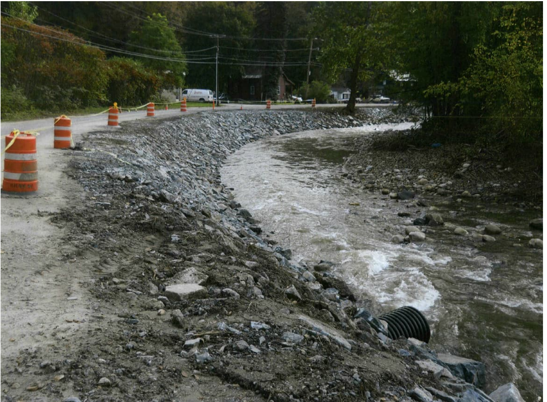
Williams Street, Brattleboro – erosion damage along sharp bend – erosion caused by deposition?
