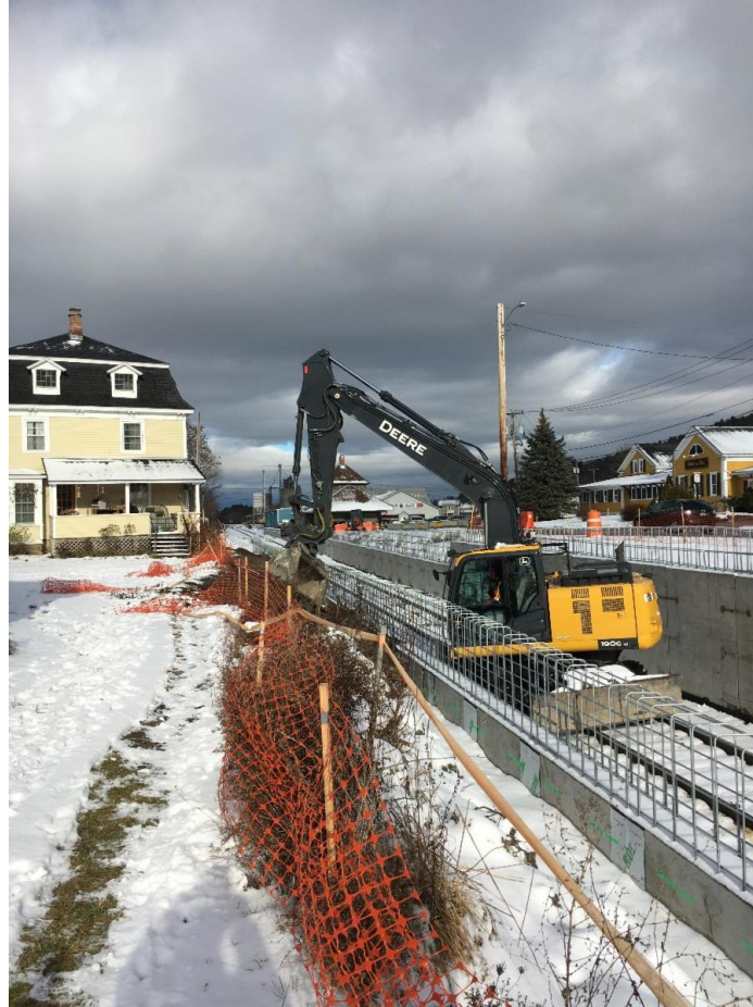
ECI stabilized the slope near Country Tire to maintain the walking path between Middle Seymour Street and the Marble Works, as shown in the above photo.
