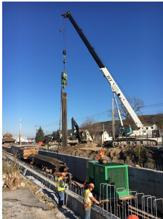
A Kubricky construction crew continued tying rebar to prepare for constructing cap walls next year.
