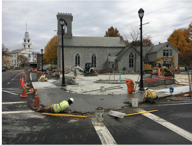
The above photo shows the Waters construction crew finishing work on the sidewalk along Triangle Park.
