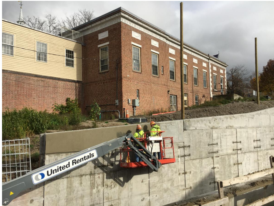
A Kubricky construction crew puts the finishing touches on the cap wall on the north end of the project site.
