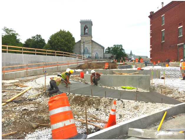
The above photo shows the Waters crew constructing the new sidewalk in Lazarus Park.
