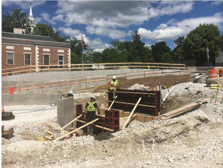
The above photo shows Waters constructing the stairs that will lead down past the labyrinth and into the Marble Works.
