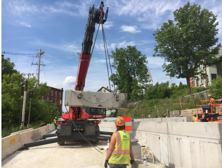
Crews removing sections of the concrete cap walls along the rail corridor south of Merchants Row.
