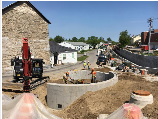
The above photo shows Kubricky grading and compacting the area surrounding the retaining wall in Lazarus Park.
