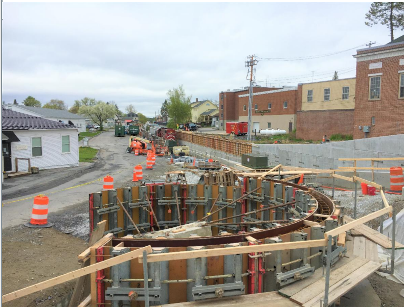
The above photo shows progress on the retaining wall in Lazarus Park.
