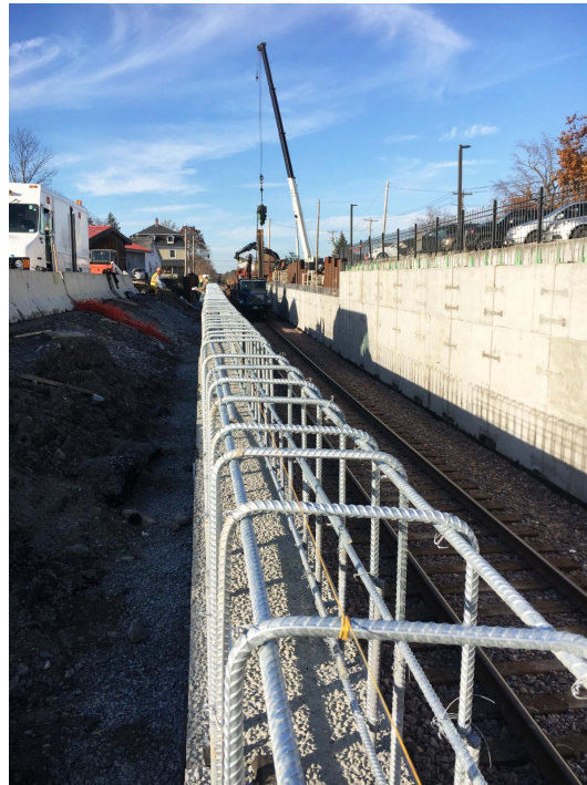
A Kubricky construction crew ties rebar to prepare for forming and pouring cap walls.
