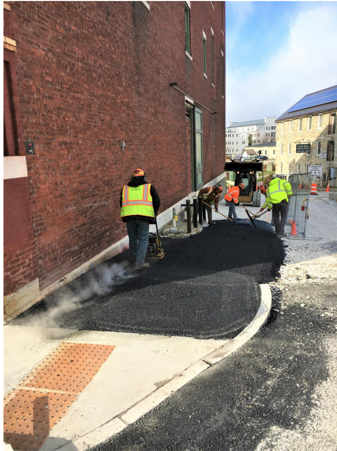
The above photo shows a Kubricky crew paving the Printer's Alley walkway.
