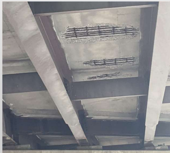
Delaminated Underside of Bridge Deck
