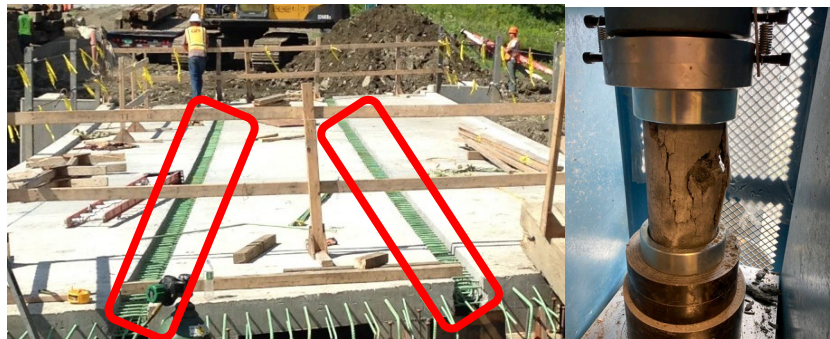
Left: VTrans ABC Connections (in red boxes) ready for RSC placement Right: RSC Mix design being tested for its compressive strength
