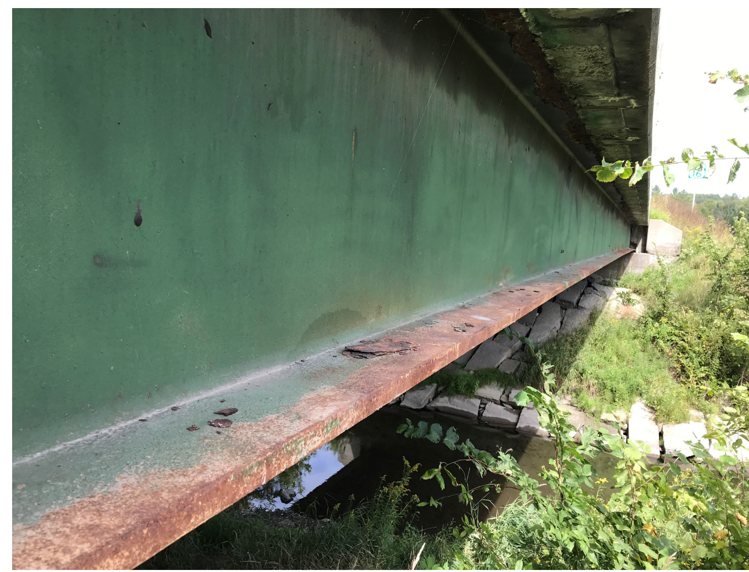
Failing paint system on bottom flange
