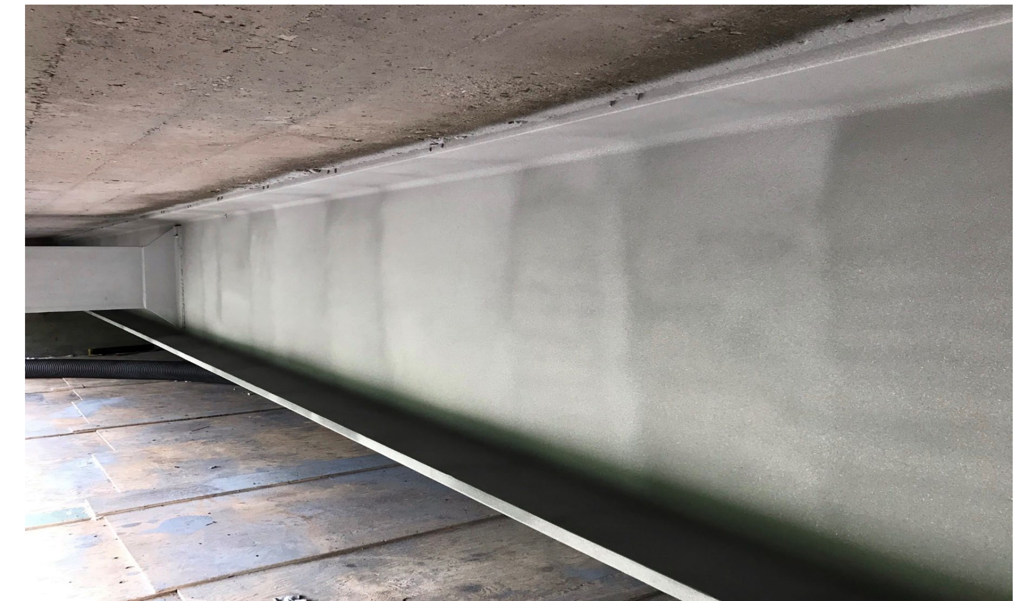
Streaks in Metalized Coating
