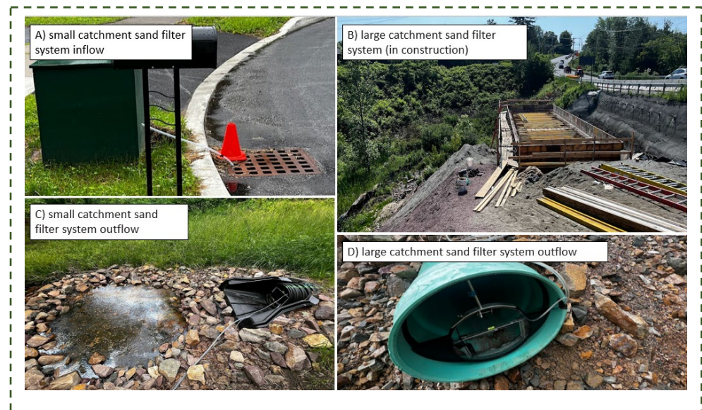
Figure 1. Photos of the small catchment and large catchment sand filter systems and associated sampling.
