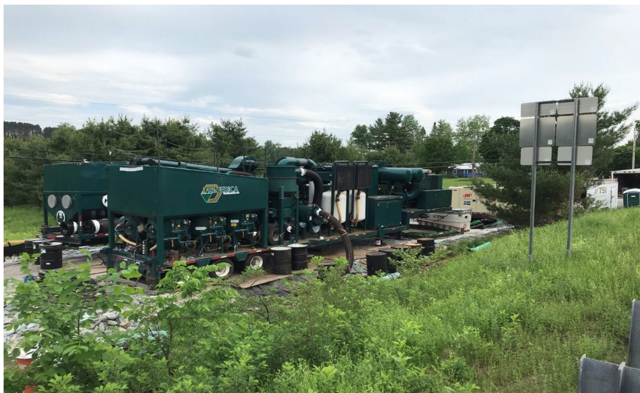
Air Filtration Equipment
