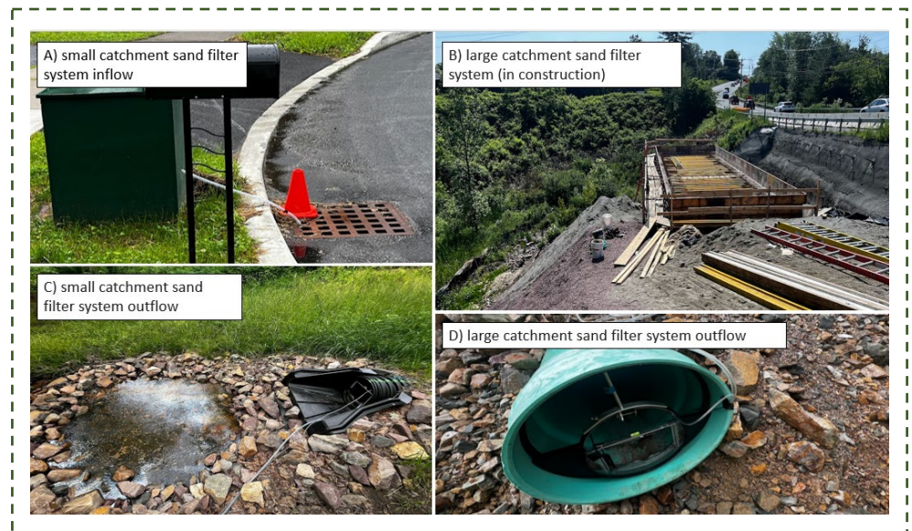
Figure 1. Photos of the small catchment and large catchment sand filter systems and associated sampling.
